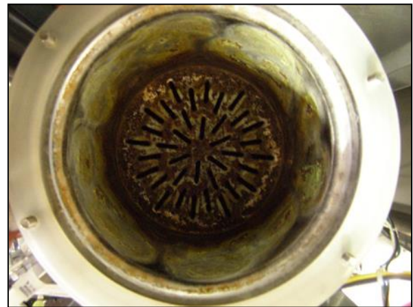
Dirty Combustion Chamber (Tft/Vmax Shown)
